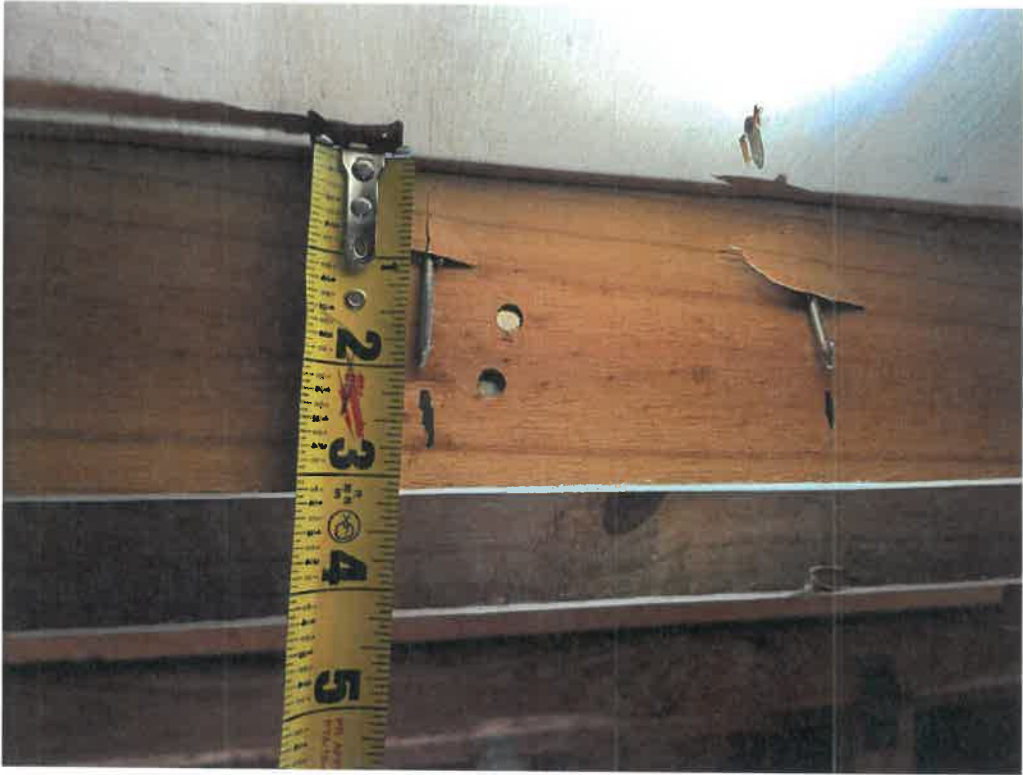
Figure 3 – Sheathing Fastener Size 8d Confirmed (Typical)
